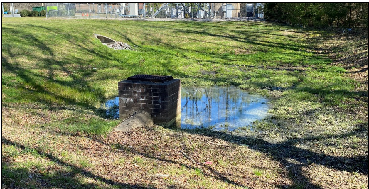
Figure 1 - A Dry Detention Basin. Recent precipitation has pooled in the forebay of this DDB, located in the eastern portion of the Greenville ETJ. Image captured by the author.
